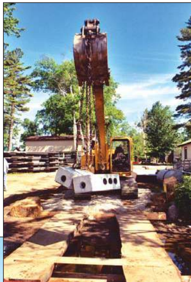
Upper photo: Loading concrete components. Lower photo: A mini-excavator helps the barge travel light.
